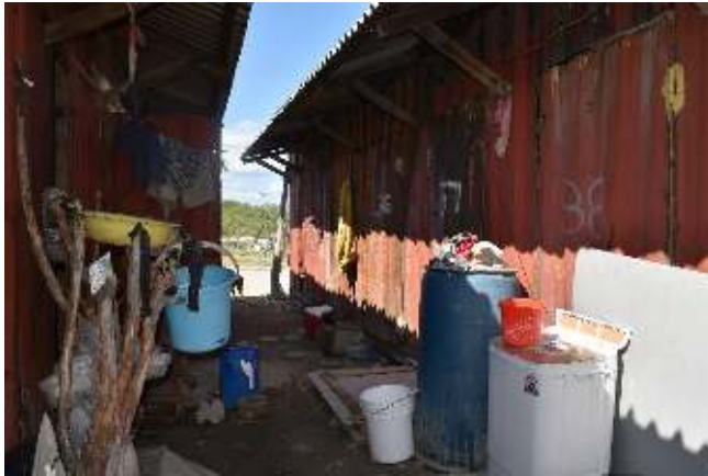
Figure 7.1: Fishers' gear lockers at the New Forum Fishing Village, which they also use as living quarters when they are staying for longer periods. In this section a fire occurred, damaging the roof of the containers. (Credit CANARI 2020)
